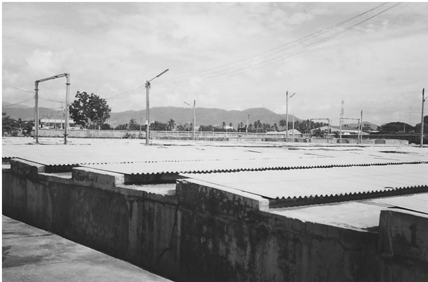
Figure 6 Fermentation pools with a corrugated tile roof. (Courtesy of Pichai Fish Sauce Co., Ltd.)
