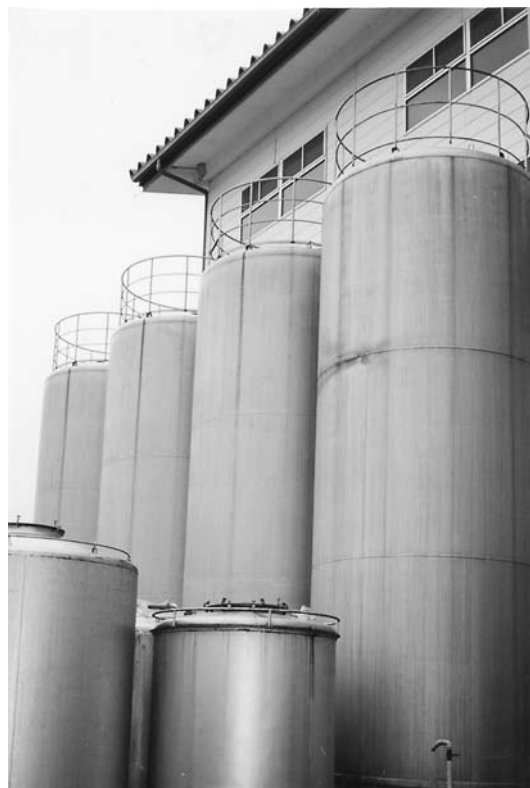
Figure 20 At some modern factories, the large-scale fermentation tanks and the storage tanks are installed outdoors.
