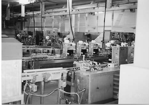
Figure 15 The interior of a filling room and an automatic filling machine. (Courtesy of Suzuyo Kogyo Co. Ltd.)
