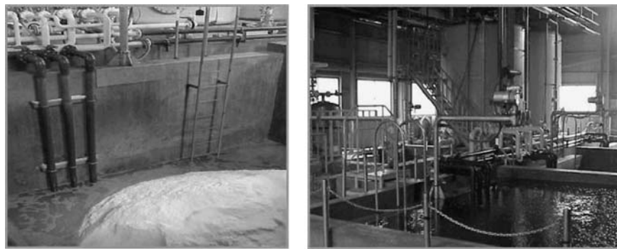
Figure 31 Brine-making facilities: left, solid salt; right, brine. (Courtesy of the Kikkoman Corporation.)
